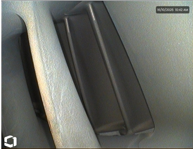
General view of Power Turbine First Stage Blades and Stator.
