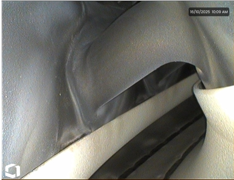
General view of CT Vane leading edge.
