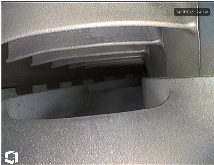
General view of CT Vane trailing edge.
